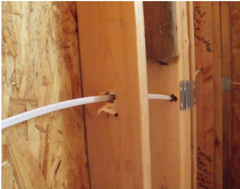
NM cable run through holes bored in the studs
