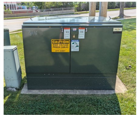
Underground service: green pad-mount transformer
