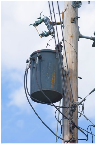
Overhead service: transformer on the pole
