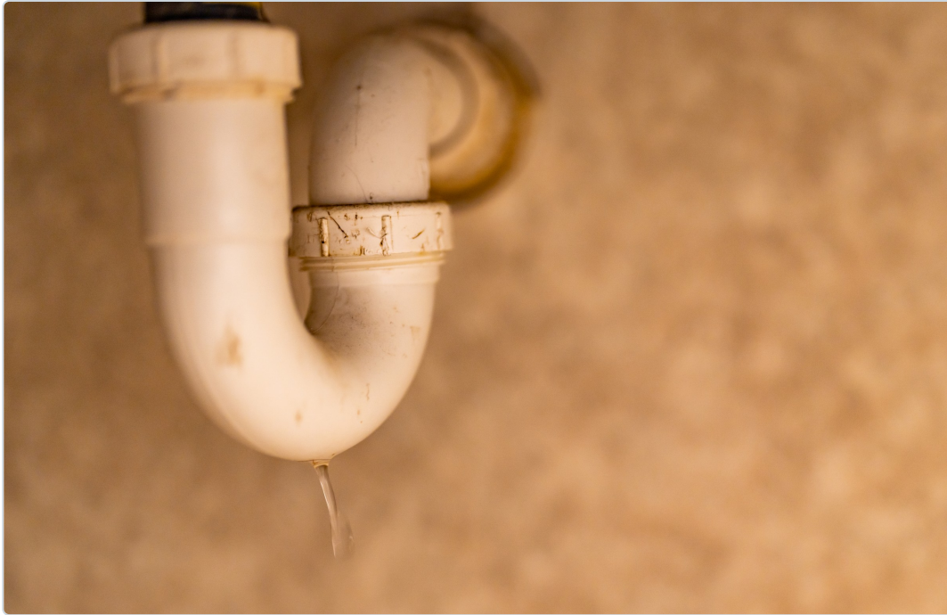
PVC P-trap under a bathroom sink. The ribbed slip-joint nuts at the top and at the trap bend hold a washer against the pipe; this one is leaking at the bottom of the trap.
