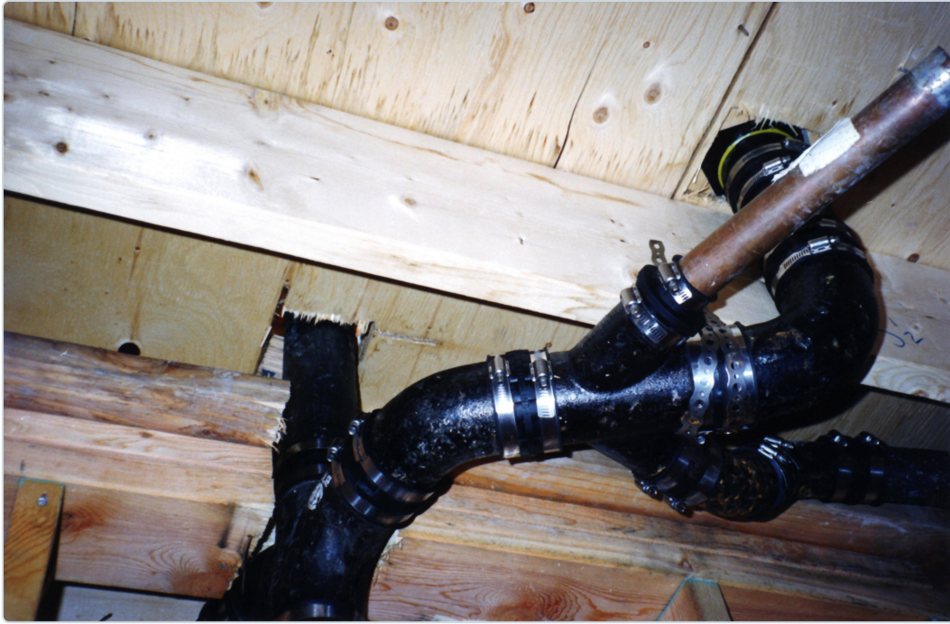
Cast iron drain pipe under a floor, joined with rubber sleeve couplings held by stainless steel bands. A copper vent pipe ties in with the same kind of coupling.
